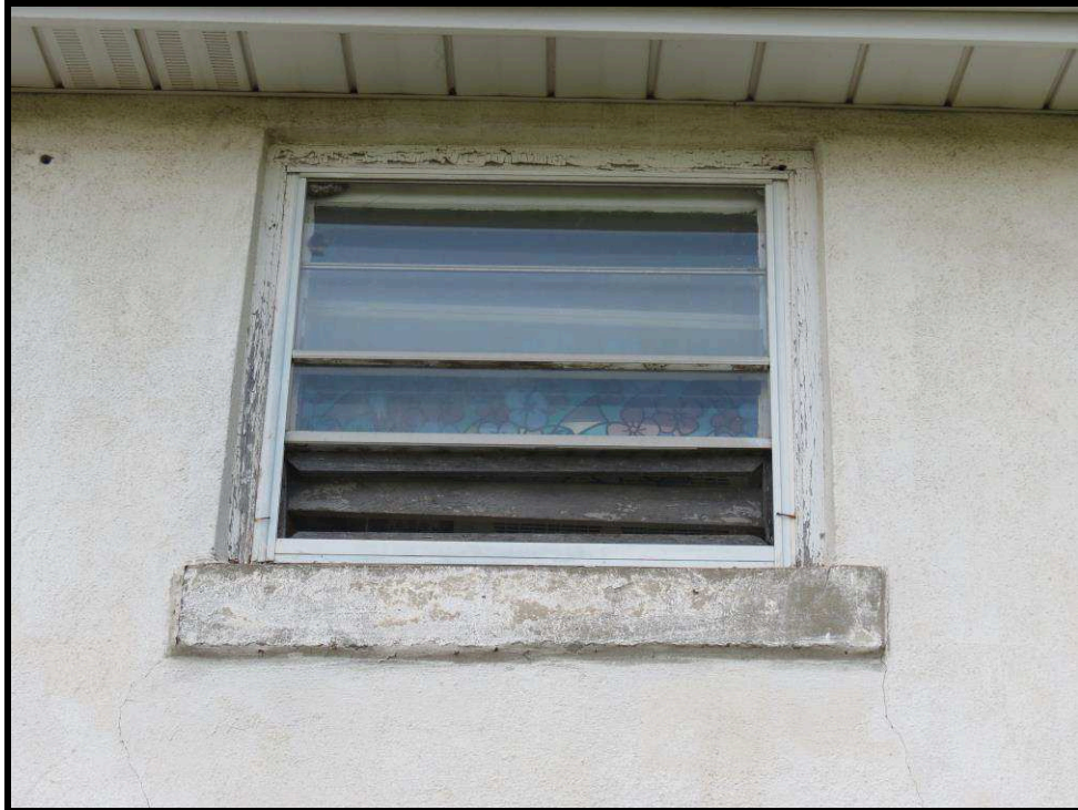
Image 20: Detail of second storey window opening (Photo taken on June 13, 2018; Facing North)
