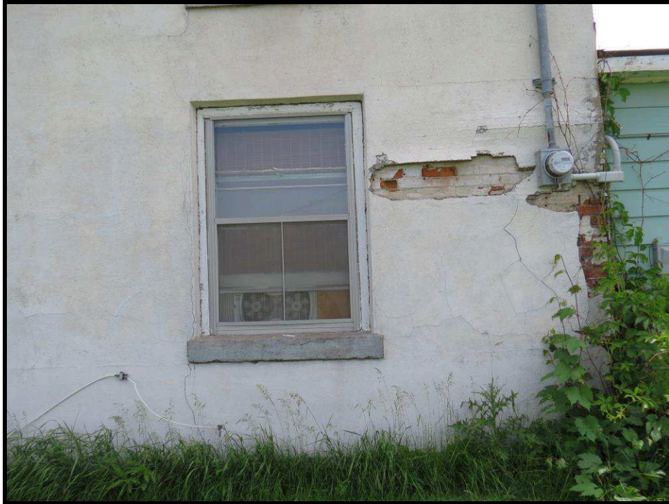
Image 28: Detail of first storey window opening (Photo taken on June 13, 2018; Facing South)
