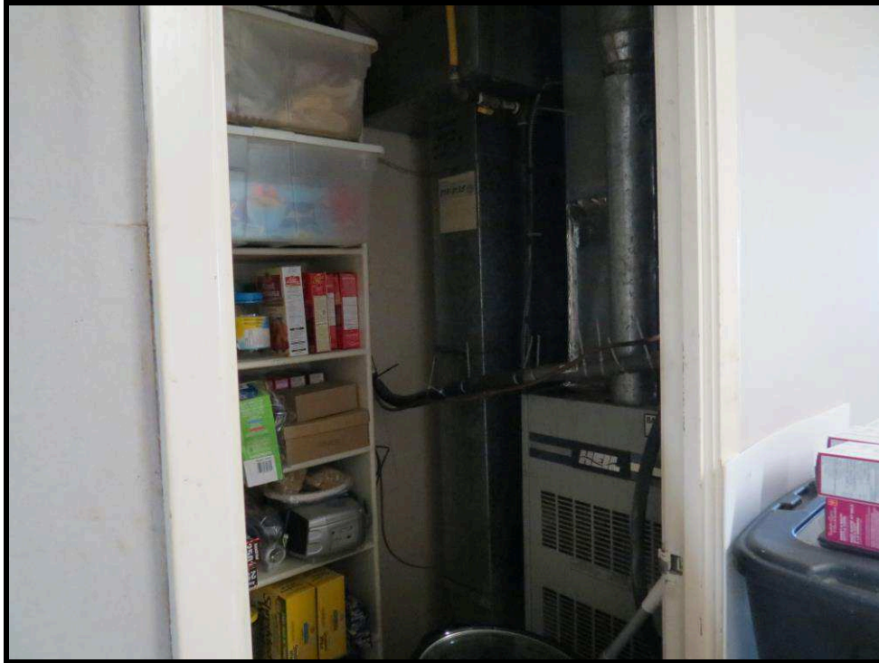
Image 39: Furnace Room (Photo taken on June 13, 2018; Facing Southeast)
