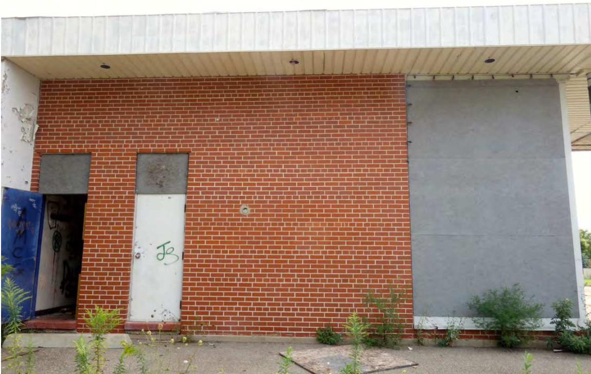
View of the north side elevation – evidence of vandalism
