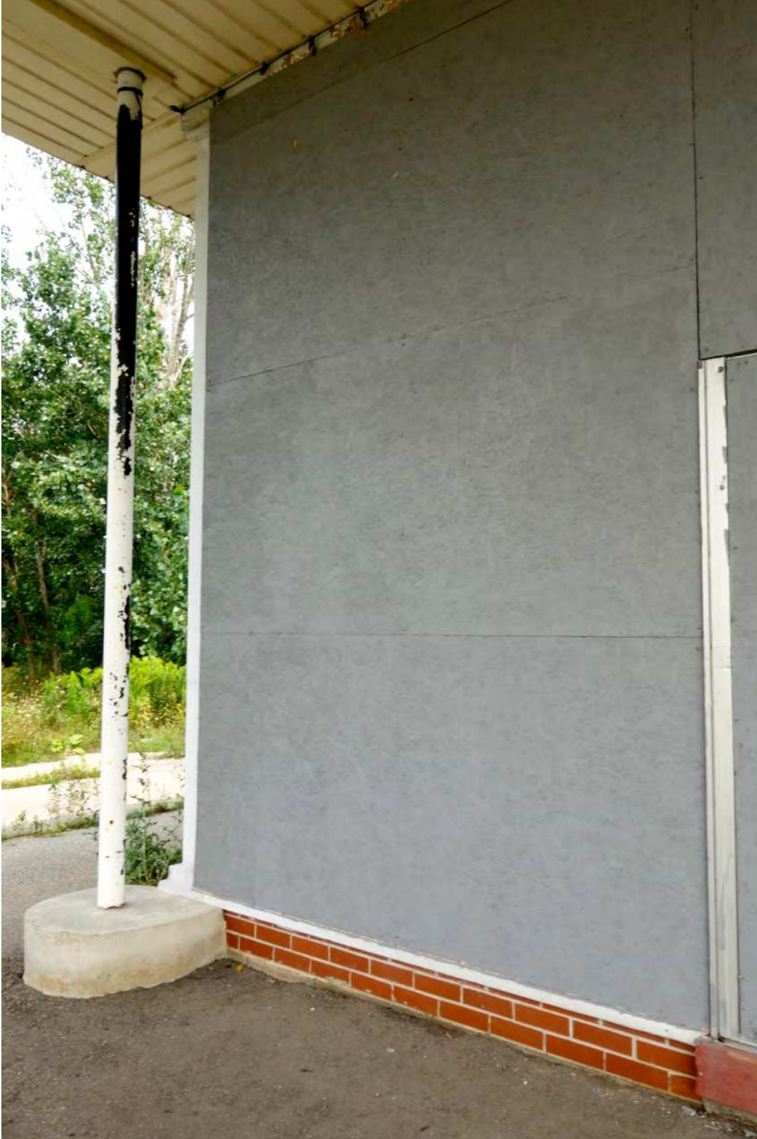
Metal posts set in concrete support the overhanging roof – vinyl cladding on soffit is not original – smooth red brick cladding – windows covered with plywood
