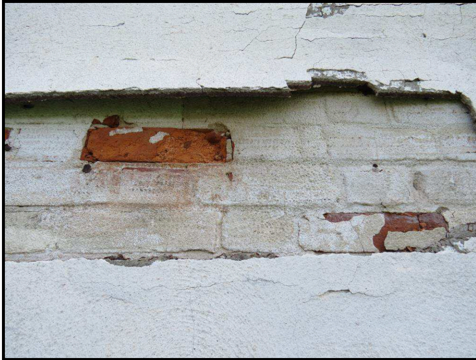
Image 29: Detail of stucco cladding over red brick structure (Photo taken on June 13, 2018; Facing South)
