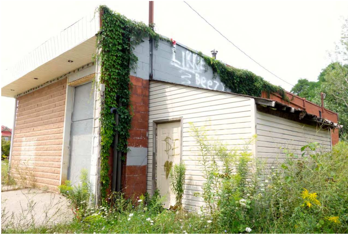
Lean-to addition at the rear with vinyl cladding – evidence of vandalism
