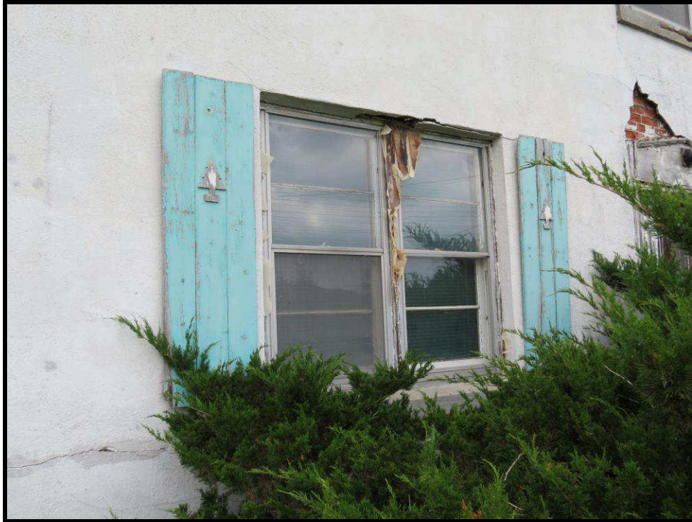
Image 12: Detail of first storey window opening (Photo taken on June 13, 2018; Facing West)
