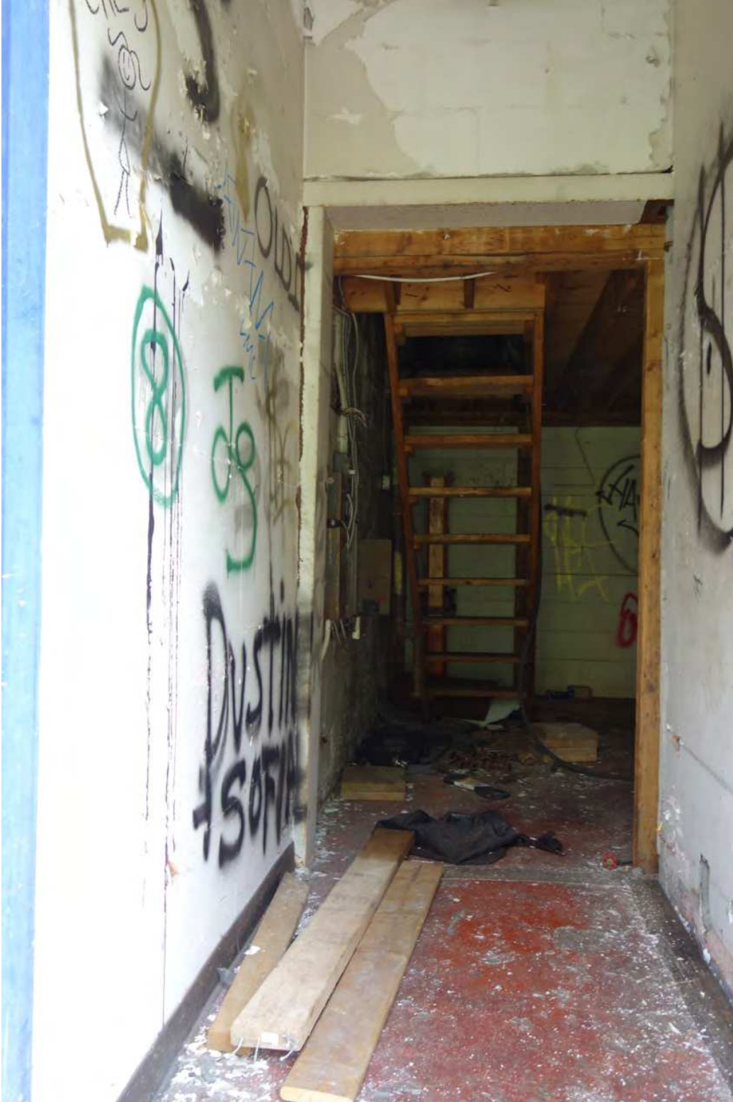
The interior was not accessible due to poor conditions – evidence of vandalism
