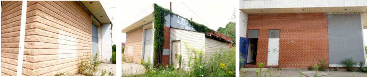
Derelict building – doors and windows are covered with plywood
