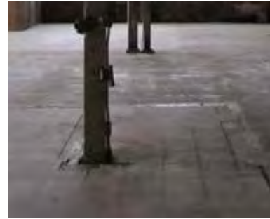
FIG 20: Interior view showing condition of cast-in-place concrete floor with linoleum tiling (ERA, 2016).
