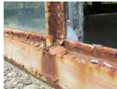
FIG 6: Detail continuous steel window on south elevation with missing pane, corrosion, and replacement silicone sealant (ERA, 2016).
