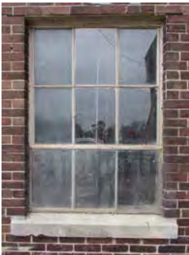
FIG 46: Single remaining original steel window on ground floor of east elevation of east courtyard (ERA, 2016).
