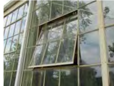
FIG 5: Continuous steel window condition on east elevation, showing horizontal pivot vent (ERA, 2016).
