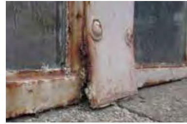
FIG 33: Detail of delaminating steel frame on north elevation at east courtyard (ERA, 2016).
