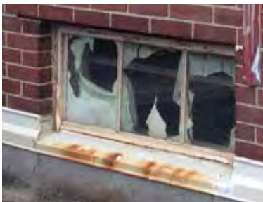
FIG 47: One of three small second floor original steel framed windows on east elevation at east courtyard. (LGA, 2016).
