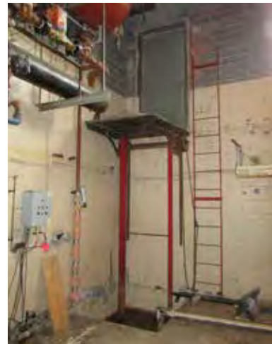
FIG 30: Mechanical lift on east wall of the Bridge in current Boiler Room (ERA, 2016).
