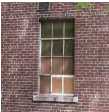
FIG 51: One of three remaining original steel frame punched windows on west elevation at west courtyard (ERA, 2016).
