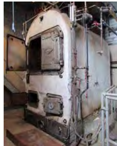
FIG 71: Original Inglis Furnace in current Boiler Room (ERA, 2016).
