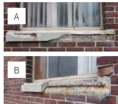
FIG 61: Sills on south elevation at east courtyard that are in an advanced state of deterioration (ERA, 2016).
