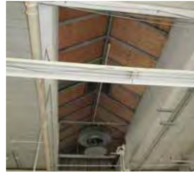
FIG 59: Large skylight in South Building showing protective boarding and missing panes (ERA, 2016).
