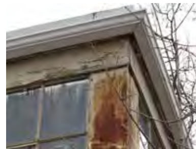
FIG 7: Detail of wood lintel with peeling paint and steel frame with corrosion at south-east corner of South Building (ERA, 2016).
