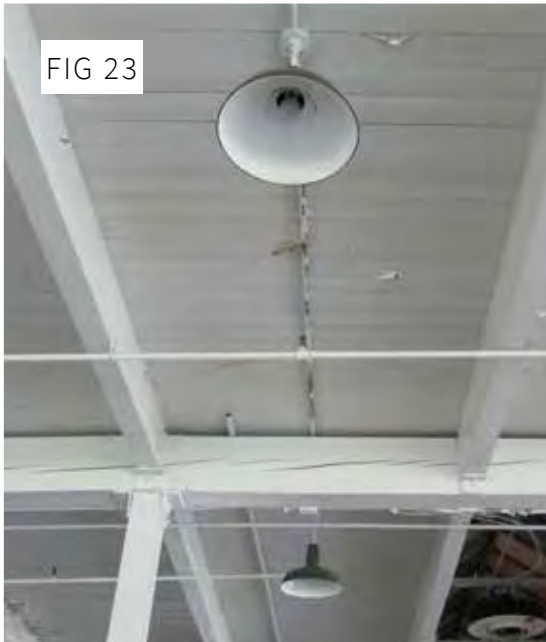
FIG 23: Condition of wood structural elements showing minor paint peeling (ERA, 2016).
