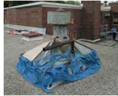
FIG 14: Condition of north-east skylight showing destructive penetration of skylight by plumbing venting stack (ERA, 2016).
