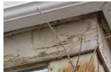
FIG 35: Detail of wood fascia showing loose/flaking lead paint (ERA, 2016).
