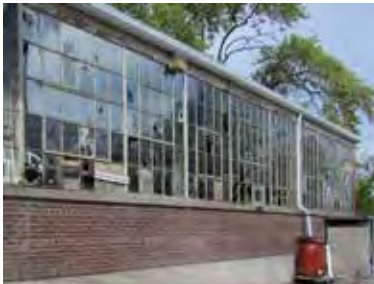
FIG 32: Condition of continuous steel windows at south-east corner of South Building showing missing and damaged glazing and corroded steel frames (ERA, 2016).
