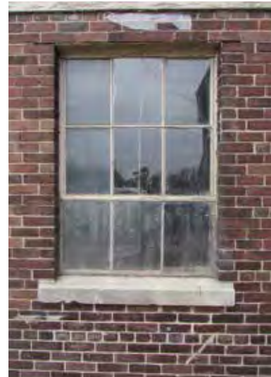
FIG 10: Original punched steel window on east elevation at east courtyard with plexiglass panes (ERA, 2016).
