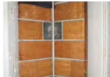
FIG 16: Detail of interior condition of large skylight showing missing lights and boarding (ERA, 2016).
