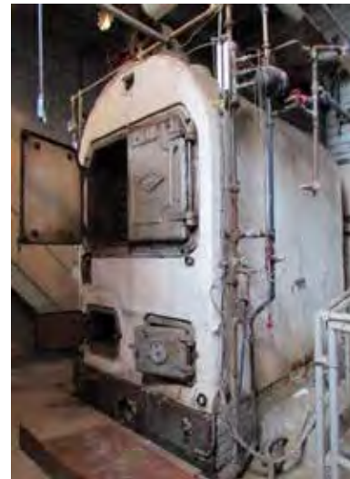
FIG 28: Original Inglis Furnace in current Boiler Room (ERA, 2016).
