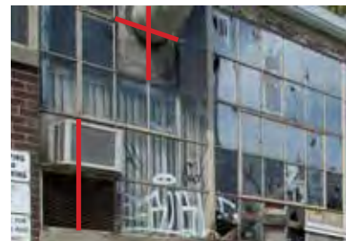
FIG 34: Area near on south elevation near south-east loading bay where the steel frame has been cut out to accommodate equipment. Missing components are annotated in red (ERA, 2016).
