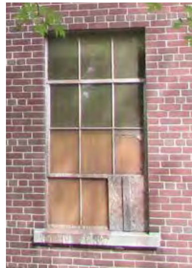
FIG 11: Original punched steel window on west elevation at west courtyard with missing/broken panes and boarding (ERA, 2016).
