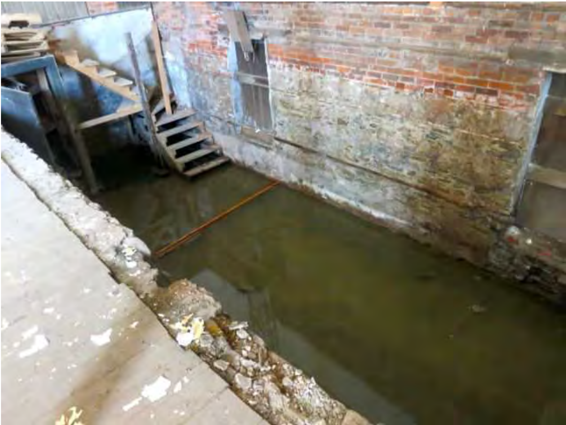
Figure 36: A large portion of the floor at the back of the ground floor is missing in an area that may have been a stage. At the time of the site visit the basement contained several feet of water.
