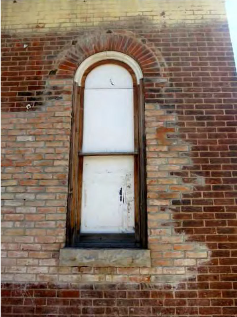
Figure 28: Poorly done restoration of the ground floor window on the main facade.
