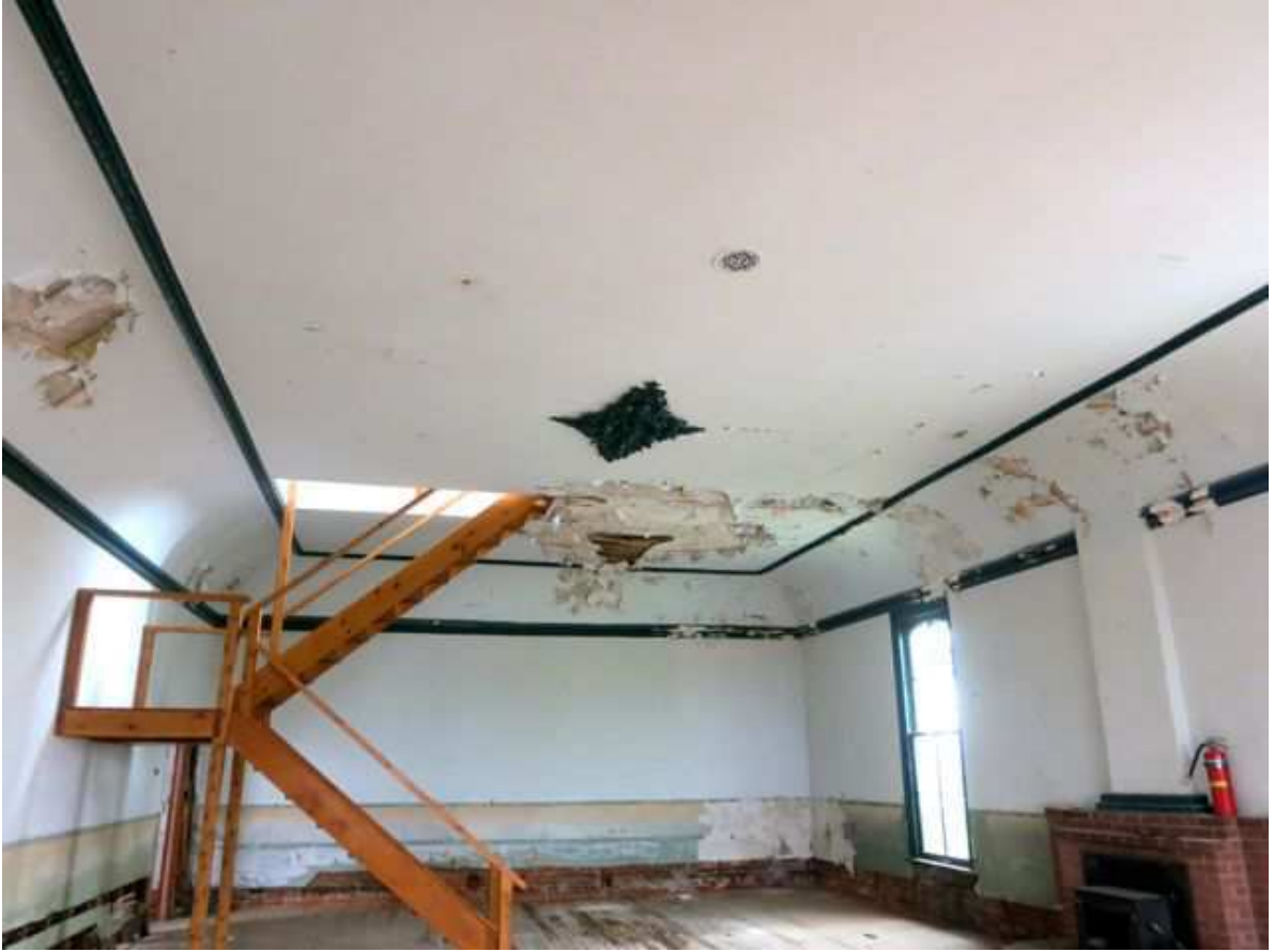
Figure 39: Large room at the rear of the 2nd floor with a coved plaster ceiling that originally served as the Odd Fellows meeting room. A modern wooden stair leads to a small loft area through an opening cut in the plaster ceiling. There is a modern brick fireplace and stove insert on the exterior wall. The plaster medallion on the ceiling matches the two plaster medallions on the first floor.
