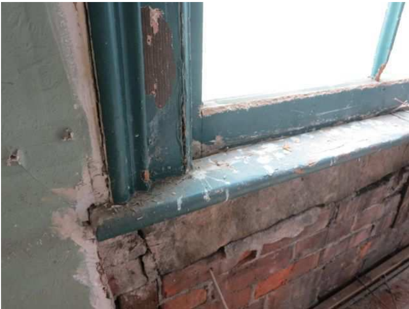
Figure 45: Detail of the original wood window sill and casing in the meeting room.
