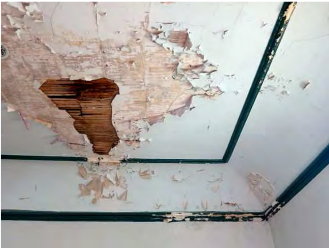
Figure 43: Detail showing an area of the plaster ceiling that has collapsed due to water damage.
