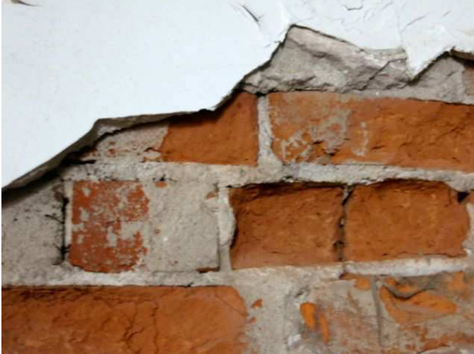
Figure 35: Lime plaster (3/4 inch thick) is applied directly to the exterior brick walls.
