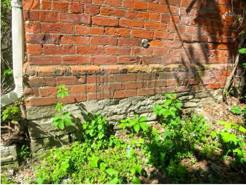
Figure 16: Rubble stone foundation with a brick apron above with a bevelled edge.
