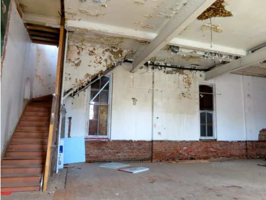
Figure 33: Ground Floor interior showing the staircase to the upper floor. Modern steel I-beams that span the interior are embedded in the exterior masonry walls.
