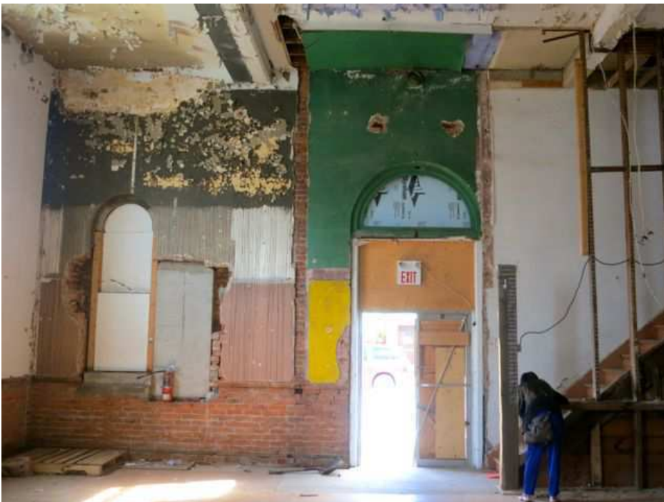
Figure 32: Ground floor interior. Front wall showing concrete block that was used to fill in an opening made for a display window.
