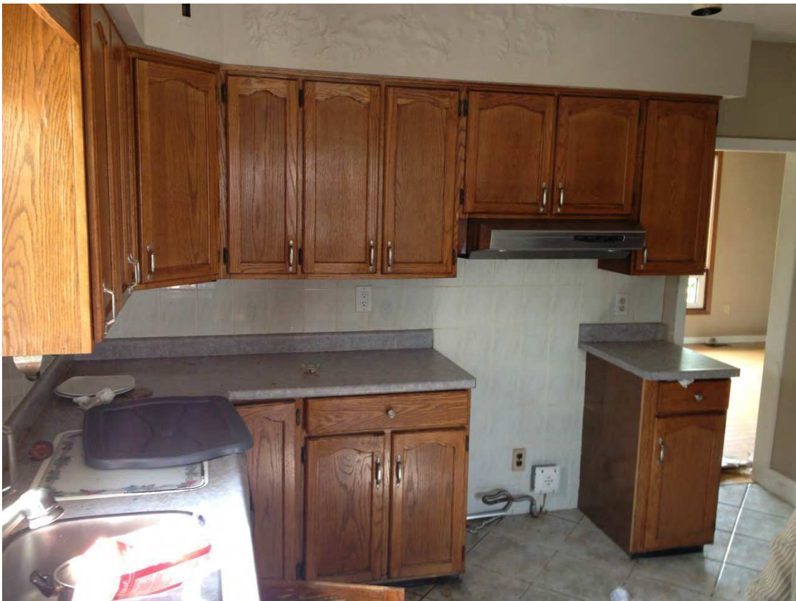
10 Queen Street South - main floor interior (note water damage above cabinets)
