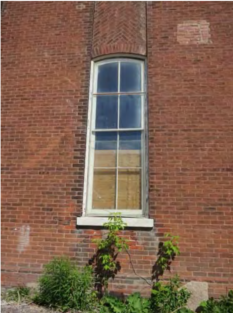
Figure 23: Large 4 over 4 wood sash window on the side elevation. Similar windows appear in the c. 1920 photo (Fig. 7) and may be original. These windows are currently not operable.
