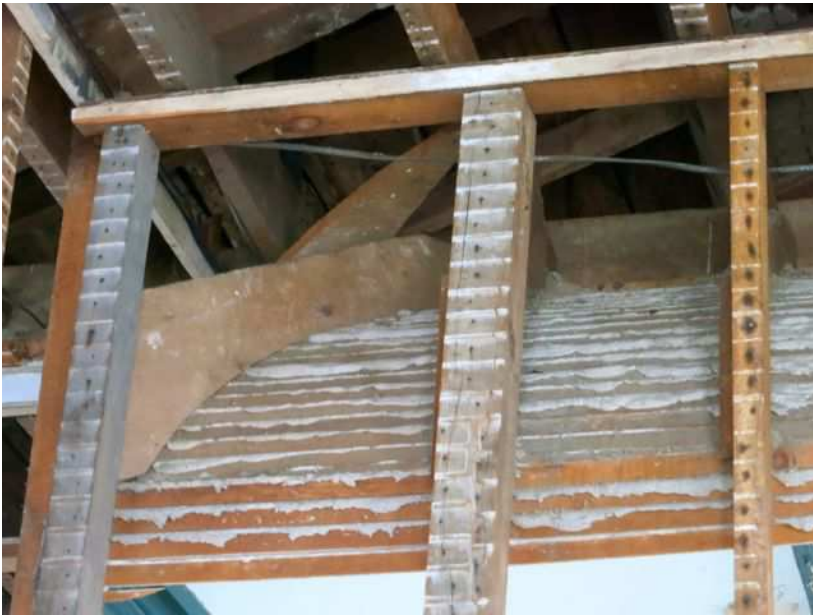
Figure 42: Detail of the lathe behind the original covered plaster ceiling in the Odd Fellows' meeting room.
