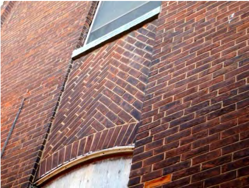
Figure 19: Decorative herring bone brickwork between the 1st and 2nd storey windows. Brick arches above the windows.
