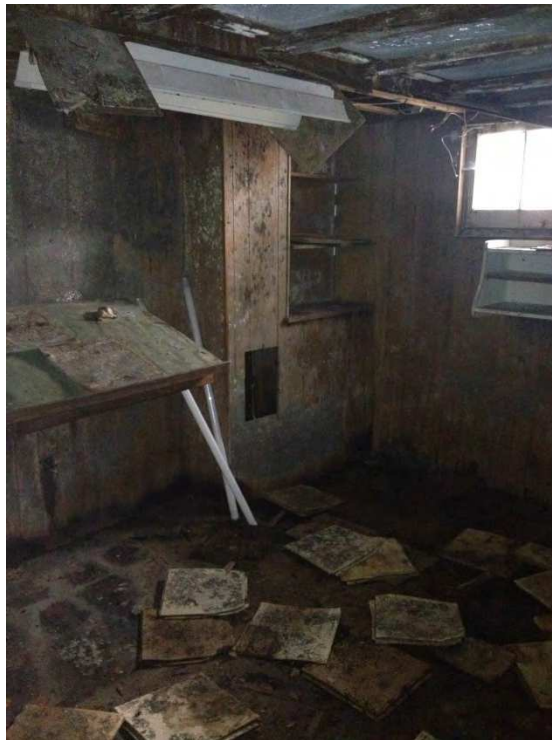
10 Queen Street South - basement interior (note extensive mould contamination)
