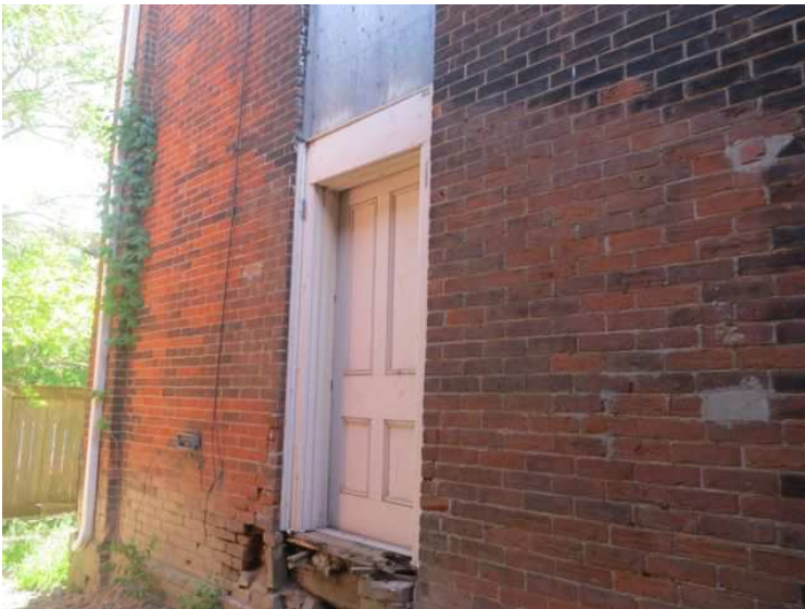
Figure 27: A wood paneled door on the side elevation at the rear. The sill has rotted and there is a large hole in the masonry below.
