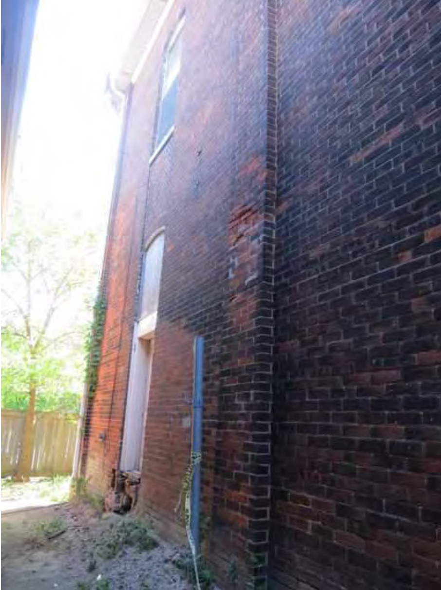
Figure 13: Side elevation in a narrow alley between the subject property and the commercial building next door. There is a large hole in the masonry below the back door sill pictured above. Brick spalling on the pier.
