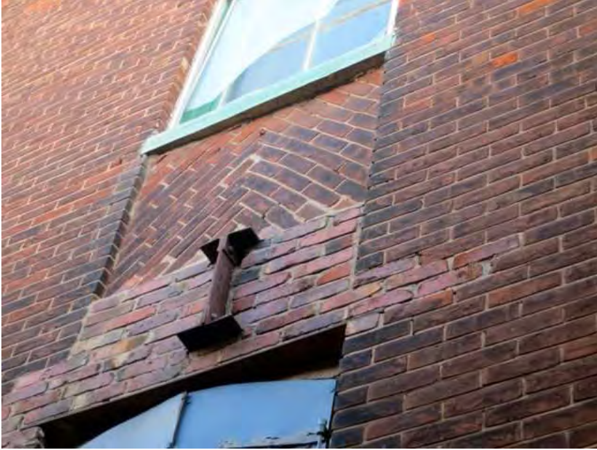
Figure 29: Three modern steel I-beams have been inserted through the exterior masonry walls
