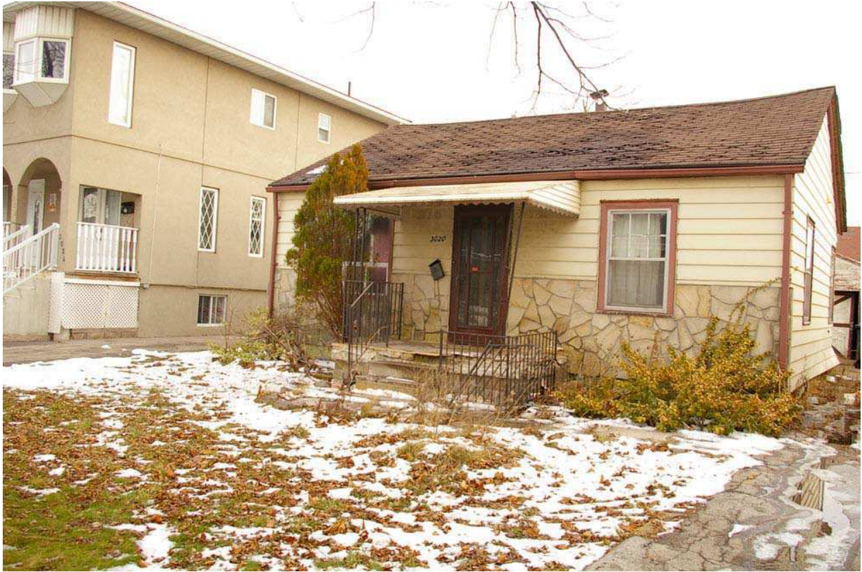
Photo 16: Existing dwelling on the subject property, looking south-east. Shows its dilapidated condition with sagging roof, concrete porch, a metal canopy, and rickety metal supports. The bedroom window to the right of the front entrance is original but the living room window has been replaced with a picture window, as better shown in the photo below. Aluminum storms were added to any original windows, probably by the first or second owners (late 50s to early 60s). Barely visible is a concrete walkway running parallel to the front façade.
