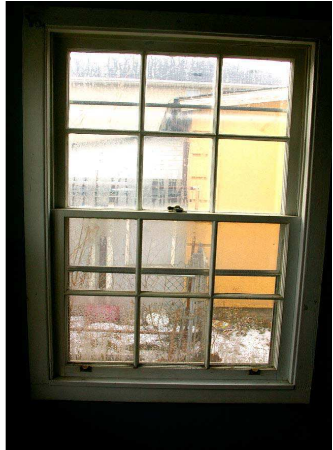
Photo 36: Close-up view of the side window, showing the wood frame and six-over-six-pane configuration of its two sashes.
