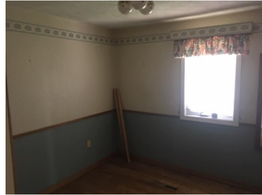
Picture 8: View of the interior of the main floor of Site Building H.
