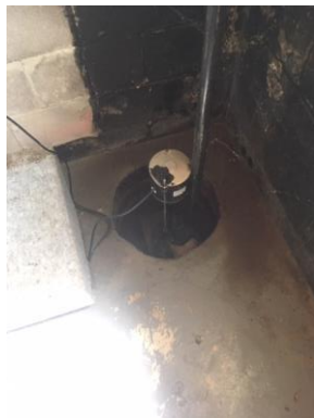
Picture 5: View of the sump in the basement of Site Building H, facing south.
