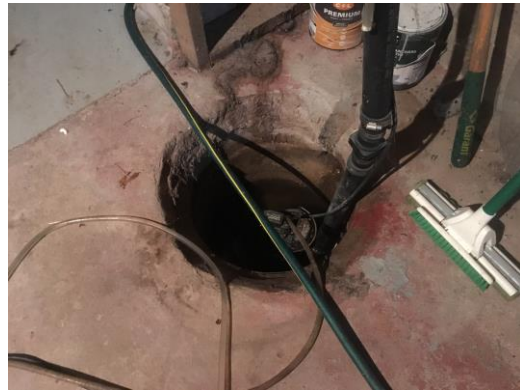
Picture 32: View of the sump located in the basement of Site Building A, facing southwest.
