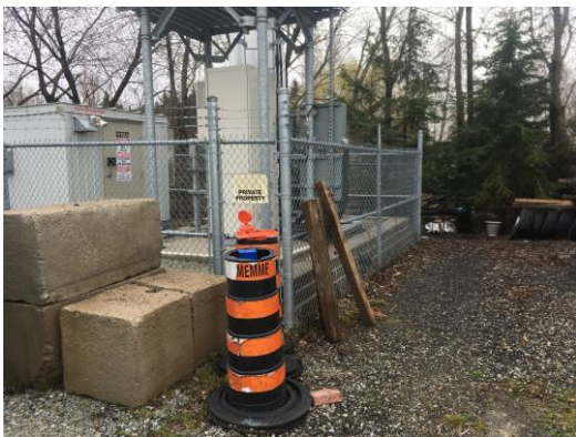
Picture 17: View of the generator and a monitoring well at the bottom of a cell tower located on the western side of Parcel E.
