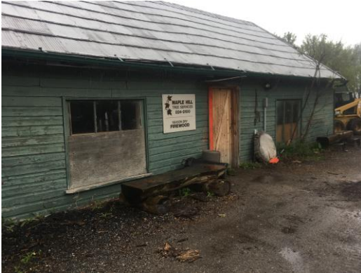
Picture 25: View of a shed used for Maple Hill Tree Services (Site Building C).
