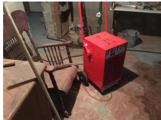
Picture 30: View of the sump and water leaks located in the basement of the Site Building A facing west.
