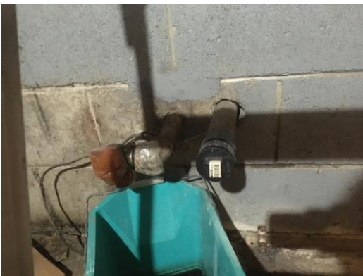
Picture 35: View of vent/fill pipe located in the basement of Site Building A, facing west.
