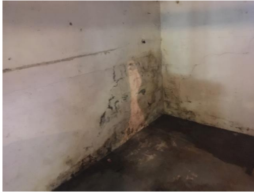
Picture 7: View of water damage in the basement of Site Building H, facing northeast.
