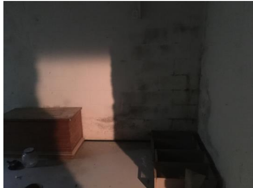
Picture 34: View of water damage in the basement of Site Building A, facing west.
