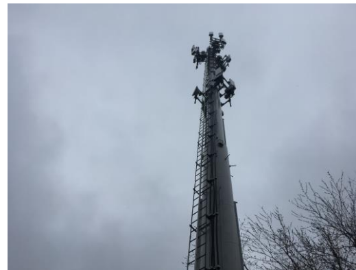
Picture 18: View of the top of the cell tower located on the western side of Parcel E.
