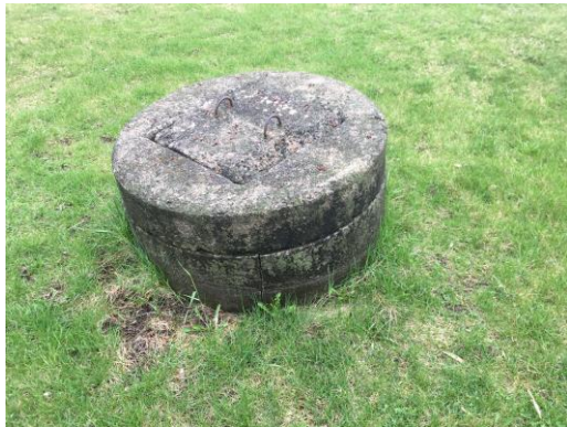
Picture 9: View of the abandoned domestic well located behind the house on Parcel E facing north.
