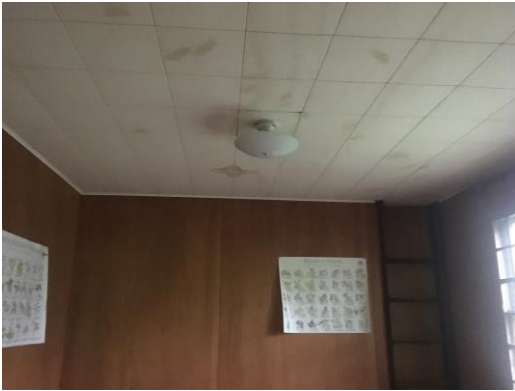
Picture 31: View of water damage on the ceiling of one of the bedrooms in Site Building A.
