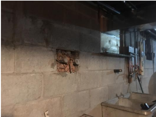
Picture 33: View of abandoned piping, located in the basement of Site Building A, facing west.
