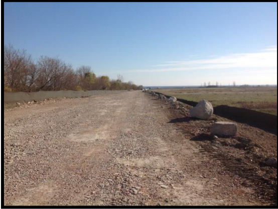
Image 5: Disturbed Lands (November 14, 2016; Facing Southeast)
