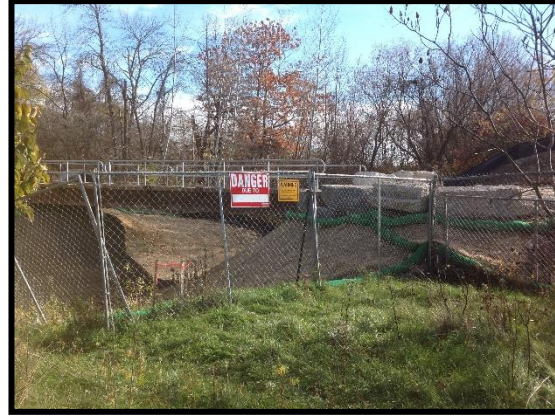
Image 6: Disturbed Lands (November 10, 2016; Facing Southeast)
