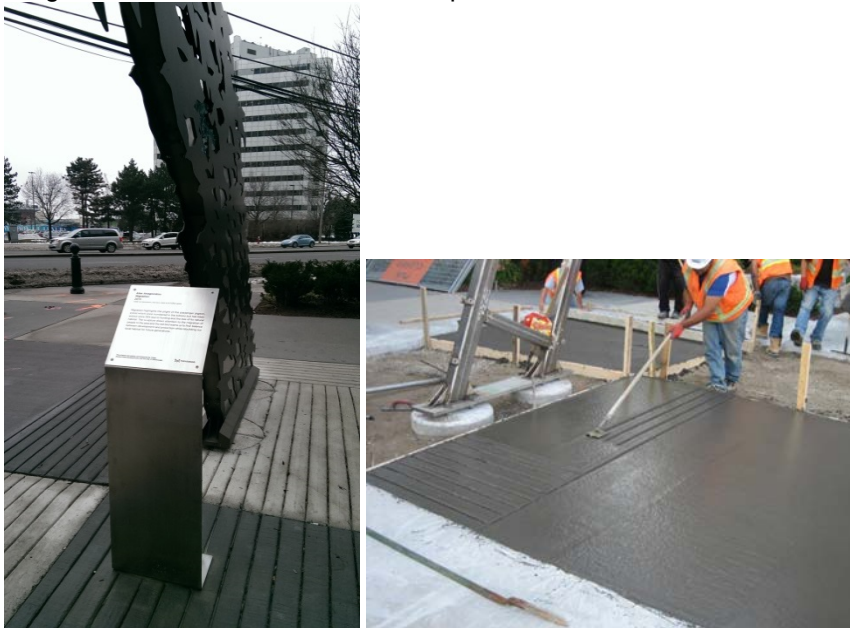
Figure 1 - Tactile warning surface around Public Art
