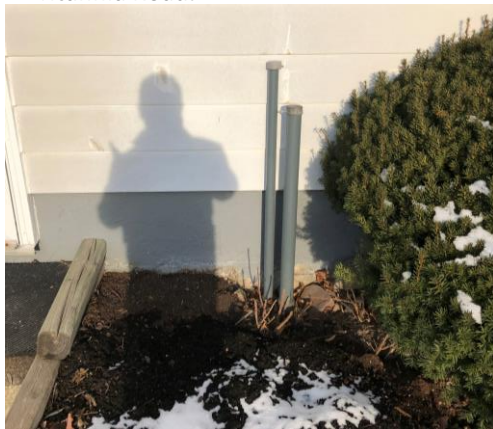
Picture 15: View of vent and fill pipes associated with basement AST in 1310 Britannia Road.
