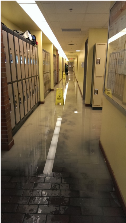
Water main break at Central Transit
