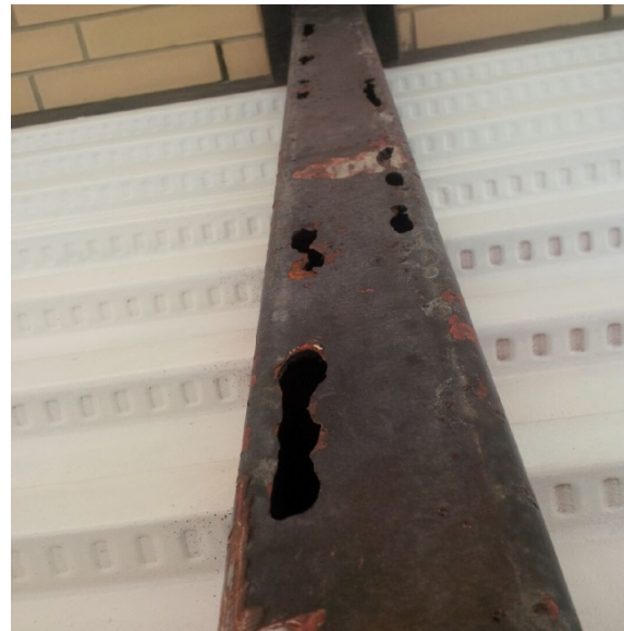
Rusting structural supports at City Hall
