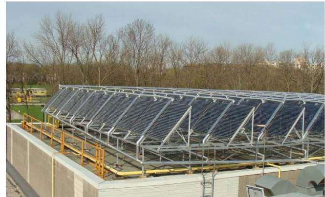
Solar Panels at Huron Park Community Centre
