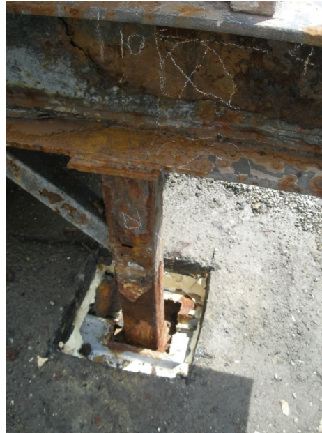
Deteriorating mechanical unit support at Iceland Arena
