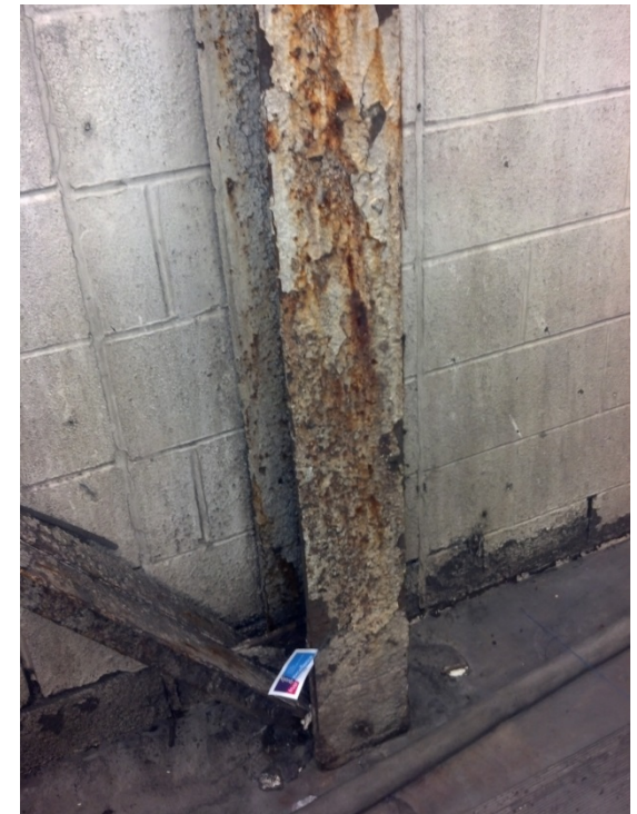
Structural steel deterioration at Central Transit wash bay
