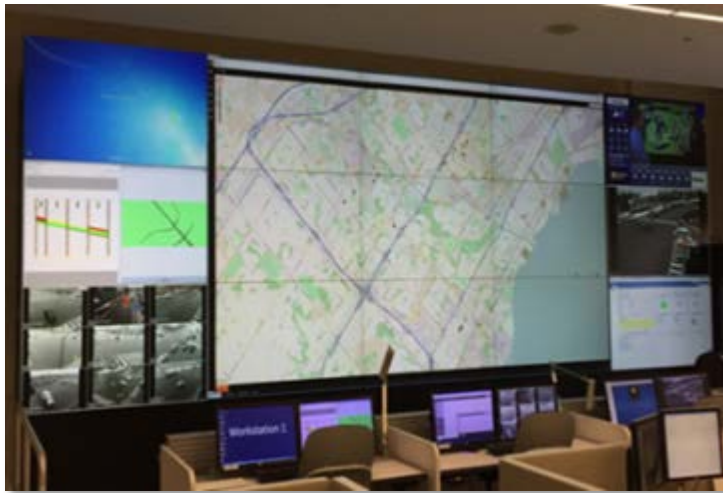
New Traffic Management Centre
