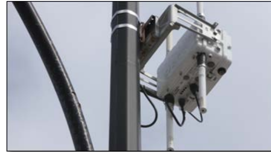
Public Wi-Fi Outdoor Access Point
