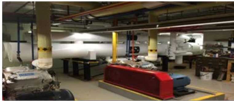
Tomken Twin Arena – Ice Plant Chiller
