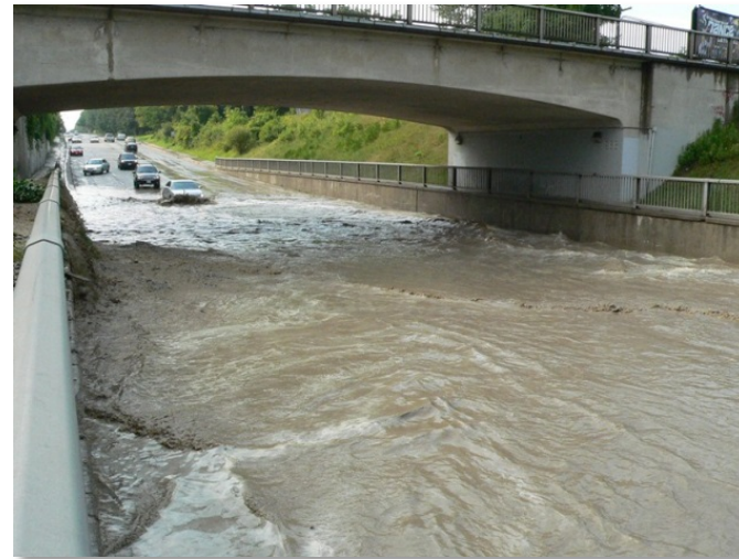
Flooding of rail underpass during an extreme storm event (source: Credit Valley Conservation)
