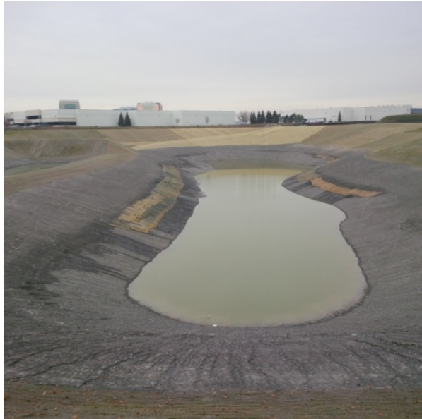
Construction of the Cooksville Creek stormwater facility located north of Matheson Boulevard West will continue into 2017
