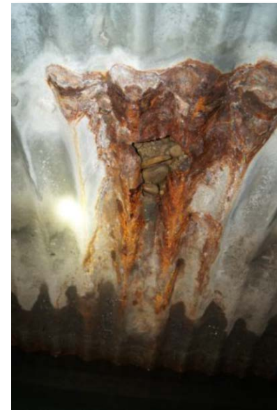
Corroded metal storm sewers require replacement
