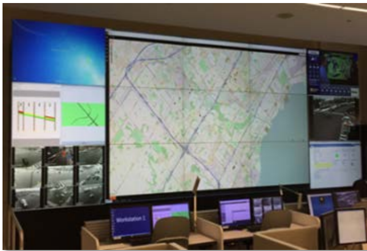
New Traffic Management Centre
