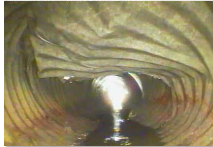
Renewal of storm sewers is a major focus of the Business Plan
