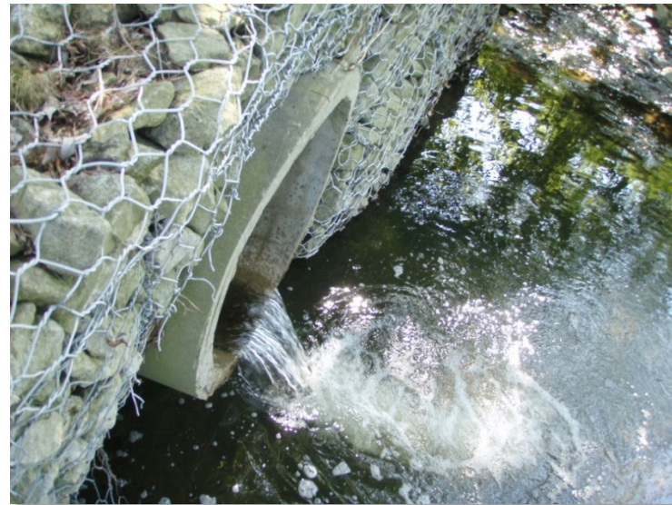
The stormwater asset management plan includes managing the City's storm sewer network effectively and efficiently
