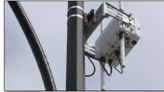
Public Wi-Fi Outdoor Access Point
