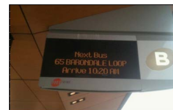
"Next Bus" Variable Message Sign
