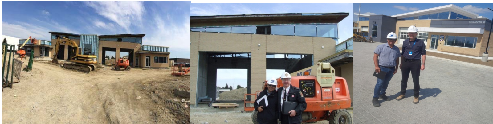
A new City Fire Station (#119) co-located with a new Peel Regional Paramedic Services Satellite Station (#11) is under construction near Pearson International Airport. This $6.4 million project is planned to be opened in the fall of 2015 and is project managed by F&PM.
