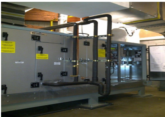
Erin Mills Twin Arena - Newly Installed dehumidification unit by F&PM Staff to provide better control of humidity levels on ice pads and building envelope.
