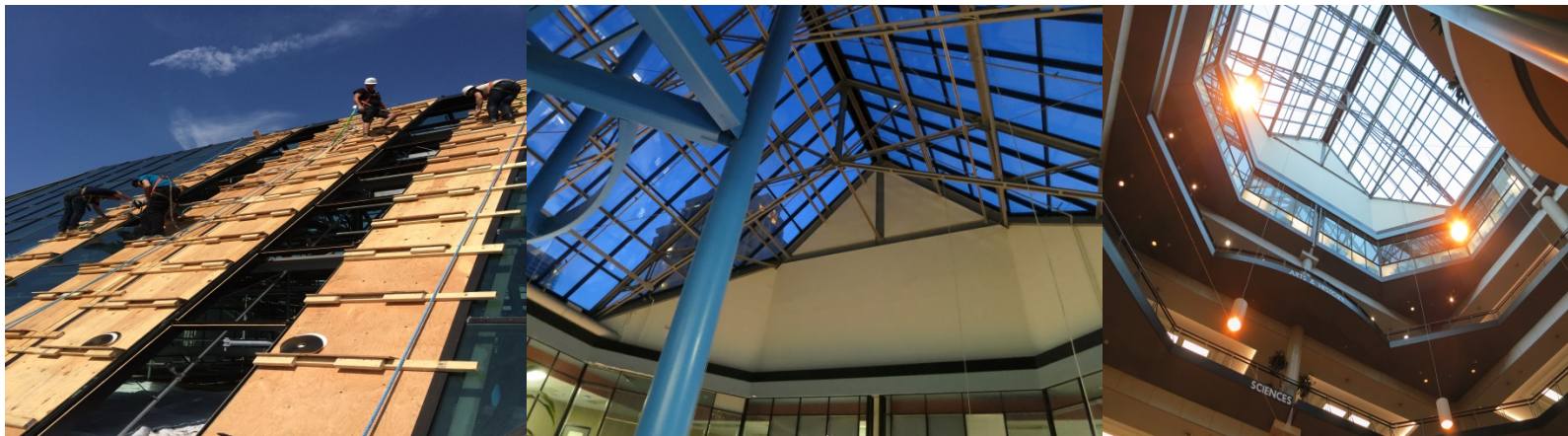
Making things brighter! F&PM led skylight lifecycle improvement project at the Central Library. The library structure is approximately 25 years old.
