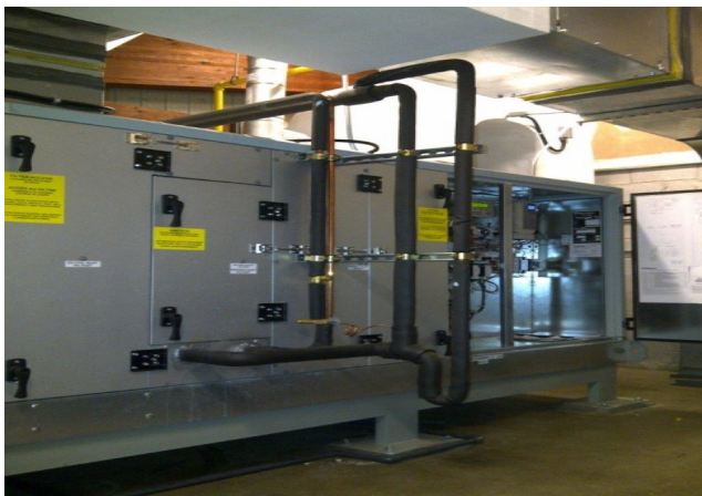
Erin Mills Twin Arena - Newly Installed dehumidification unit by F&PM Staff to provide better control of humidity levels on ice pads and building envelope.
