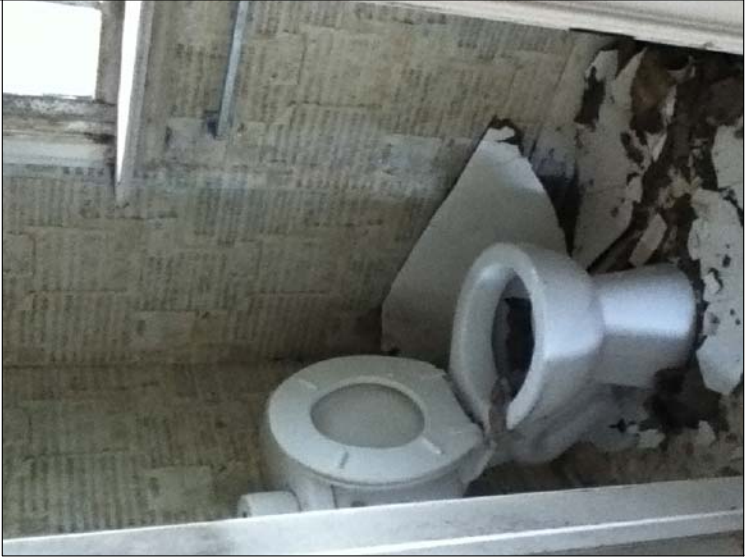
2-STORY HOME - POWDER ROOM - NOTE WATER DAMAGE
