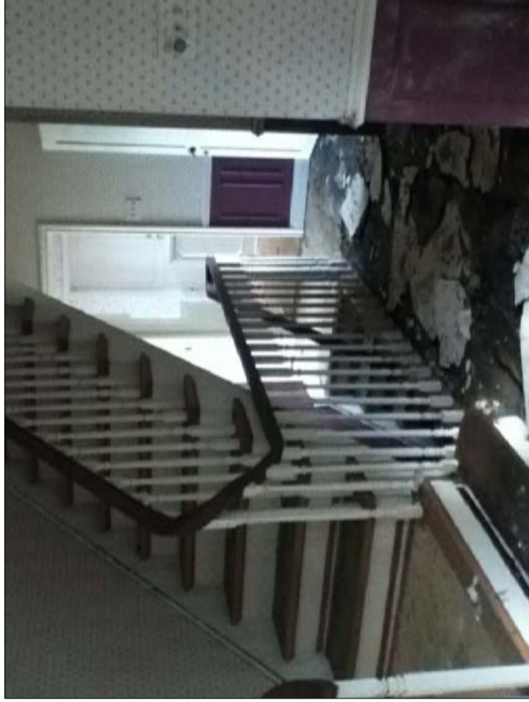
2-STOREY HOME - HALL - NOTE DAMAGE FROM WATER LEAKAGE
