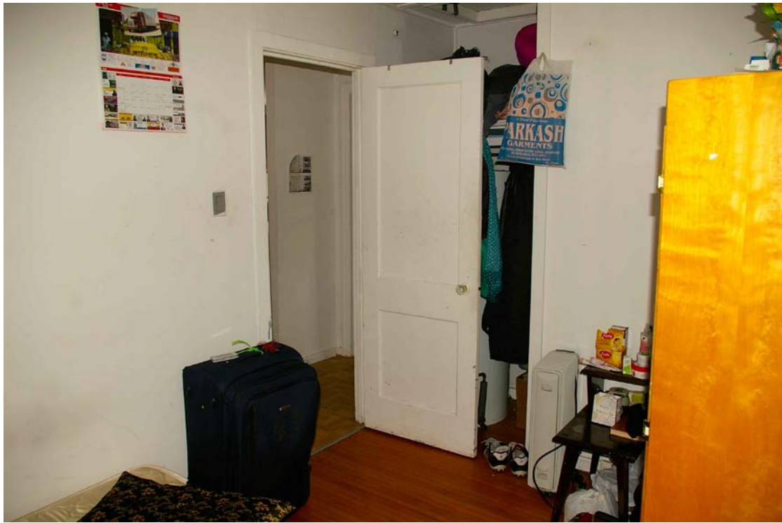
Photo 40: Rear bedroom looking through the doorway into the hallway. Front wall and doorway to the closet appear to have been removed when a replacement water heater was installed (partially visible behind the door).
