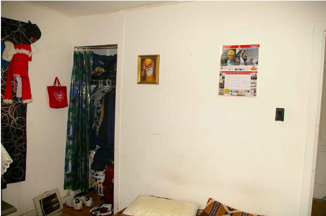
Photo 43: Back wall of the front bedroom with the doorway partially visible on the right and an original closet (with door removed).
