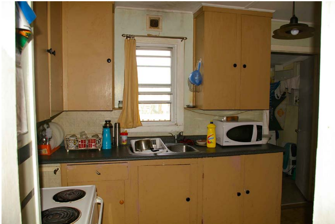
Photo 35: Rear wall of the kitchen, kitchen window and doorway to the laundry room on the right. It is surmised that the water heater was originally located in the corner beside the wall shared with the bathroom and when relocated the countertop was extended into this space.
