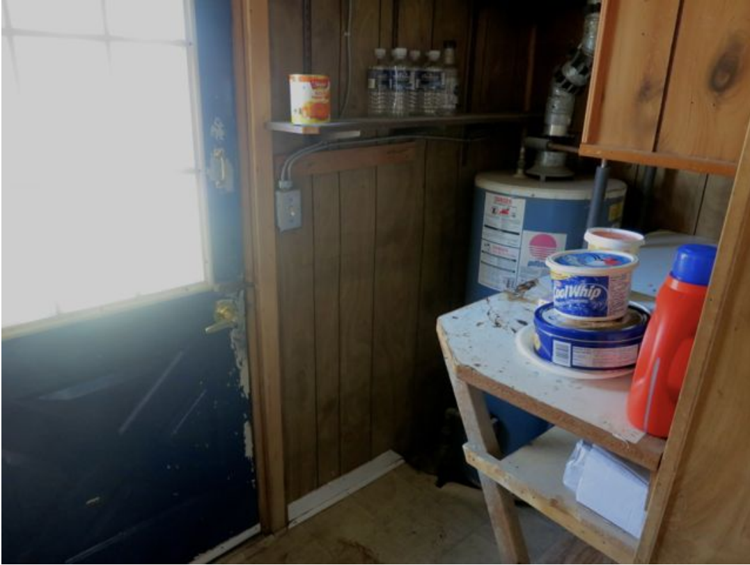
Figure 21: 3032 Churchill Avenue, the water heater is located in the back entry vestibule
