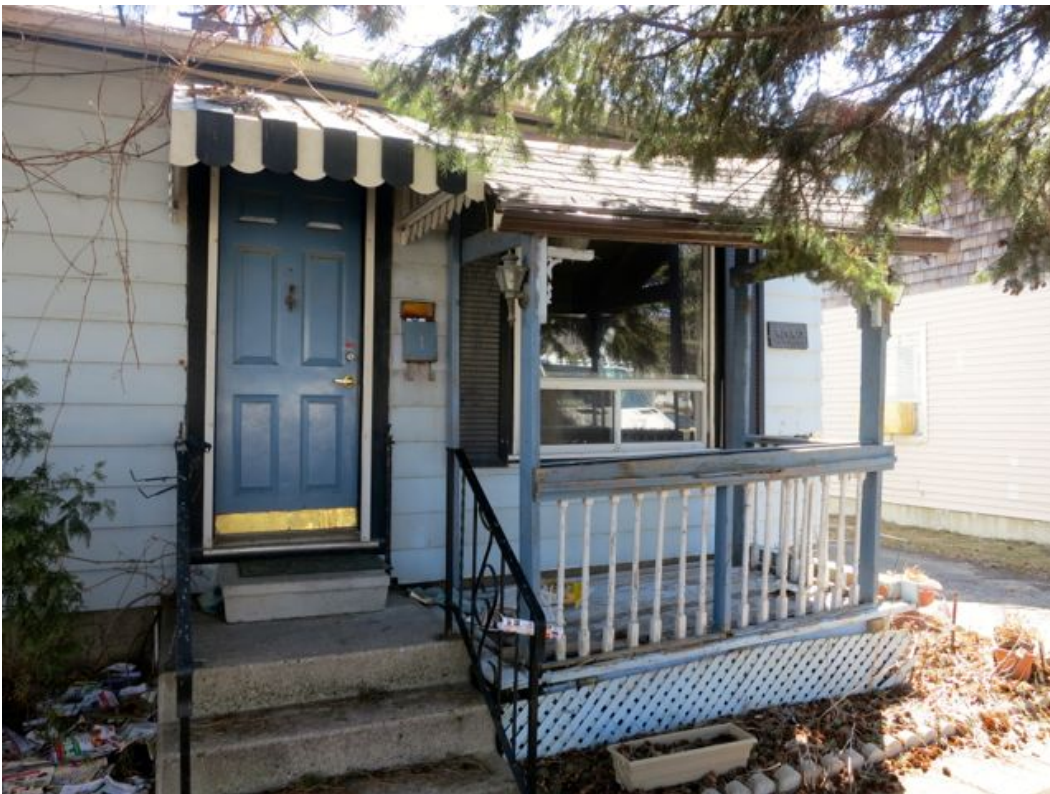
Figure 12: 3032 Churchill Avenue, front entrance. Changes to the original design include the metal handrails, metal canopy, wooden porch, paneled front door, picture window and aluminum siding.
