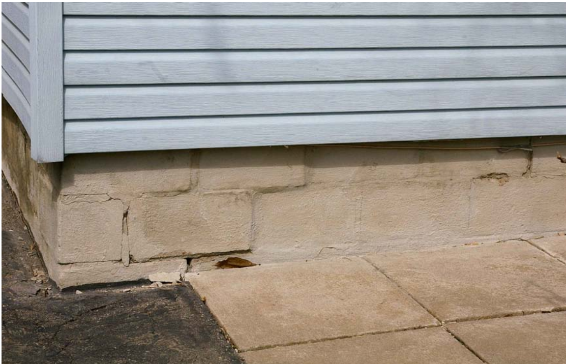
Photo 17: Detail of concrete block foundation and vinyl siding on the front facade at the junction of the asphalt driveway and concrete paving stone walkway to the front porch.
