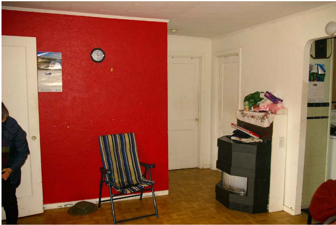
Photo 30: Living room looking towards the short hallway to the rear bedroom and bathroom, with the archway to the kitchen on the right. The existing wood-burning stove stands in the same location as the original coal- or wood-burning stove, with the chimney flue directly behind in the kitchen.
