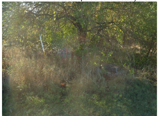
Plate 22: View S at buried gas pipeline and utility access cover at the intersection of Sheridan Park Drive and the east leg of Speakman Drive.
