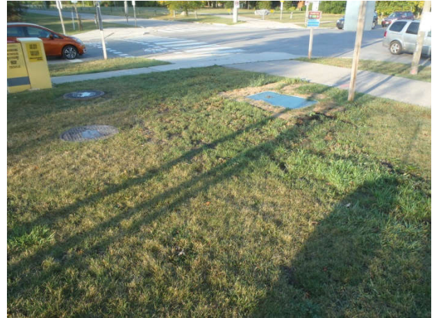
Plate 24: View W at disturbance due to buried utilities at the east side of the intersection of Sheridan Park Drive and the east leg of Speakman Drive.
