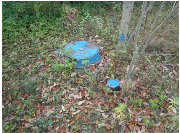
Plate 18: View SE utility access covers in the eastern portion of the study area.
