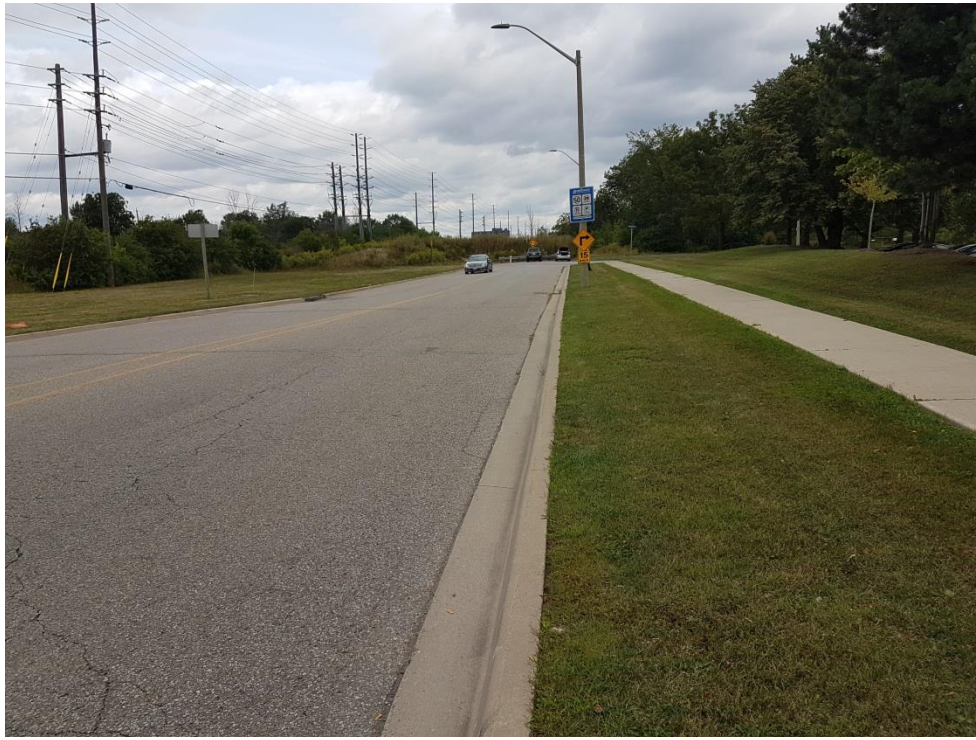
Photograph 7: Random Minor Crack at west end of Sheridan Park Drive.
