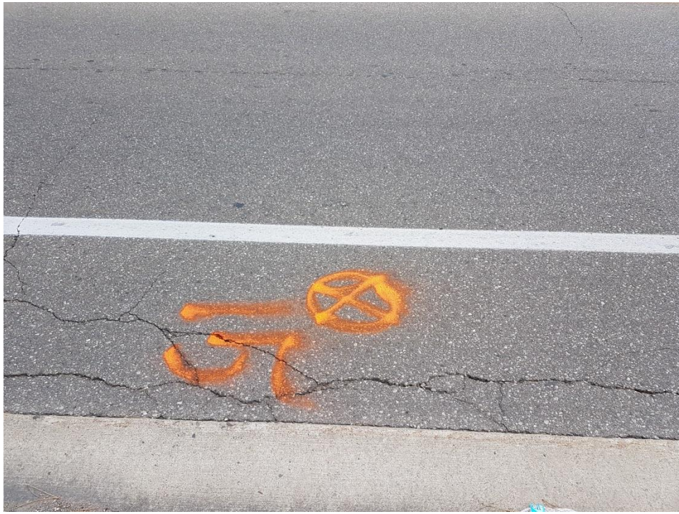
Photograph 11: Wheel track crack at north and longitudinal crack along curblines near BH15.
