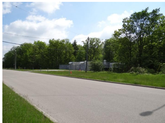
Plate 6: Electrical transformer station on the south of Sheridan Park Drive, looking southeast.
