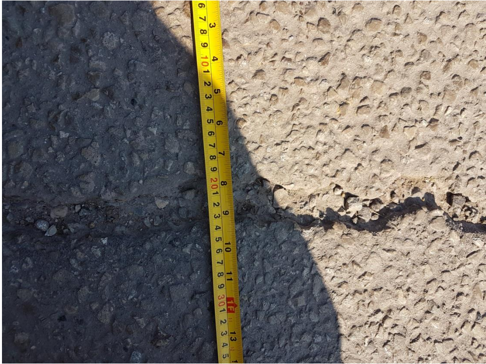
Photograph 2: Moderate longitudinal crack segregating and coarse aggregate loss.
