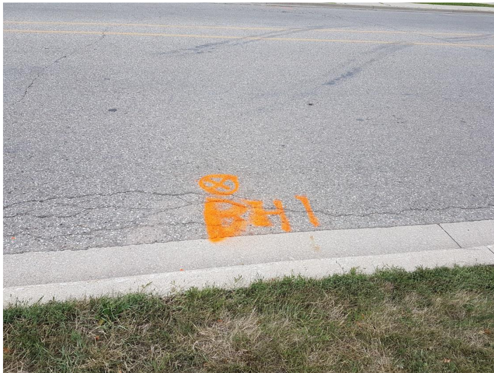
Photograph 6: Longitudinal and transverse cracks near BH1.
