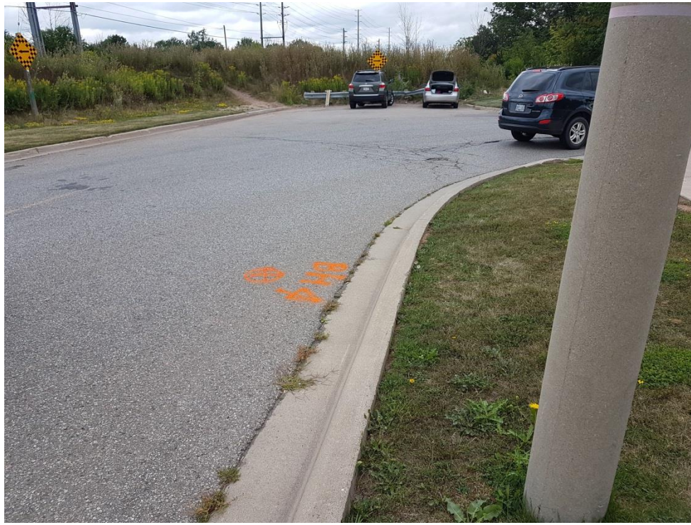
Photograph 5: Distortion from frost heaving near BH4.
