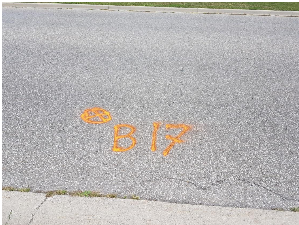
Photograph 12: Crack along curblines near BH17.
