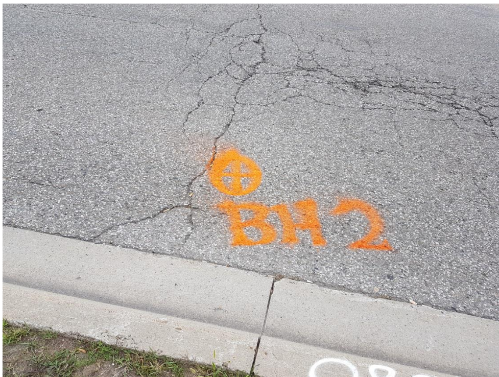
Photograph 4: Severe distortion from frost heaving near BH2.
