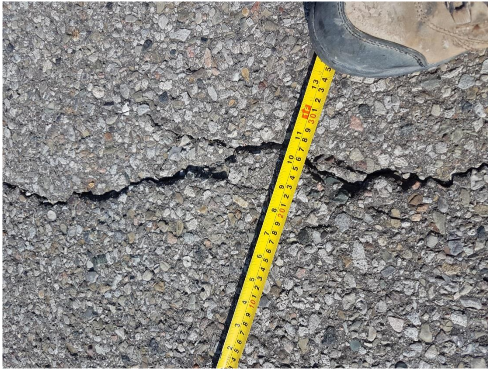
Photograph 13: Coarse aggregate loss, moderate longitudinal cracking.
