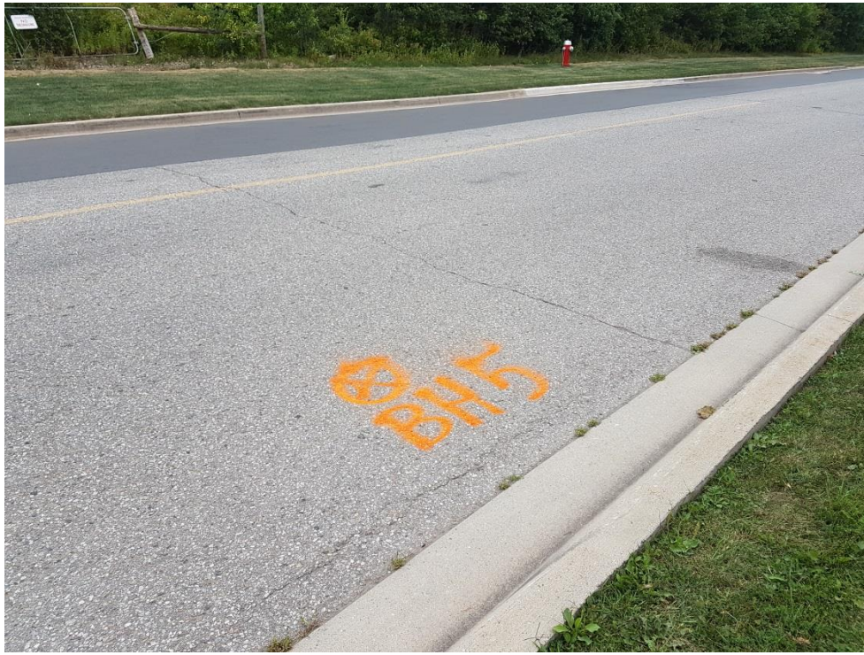
Photograph 9: Slight longitudinal and transverse crack near BH5 on Speakman Drive.
