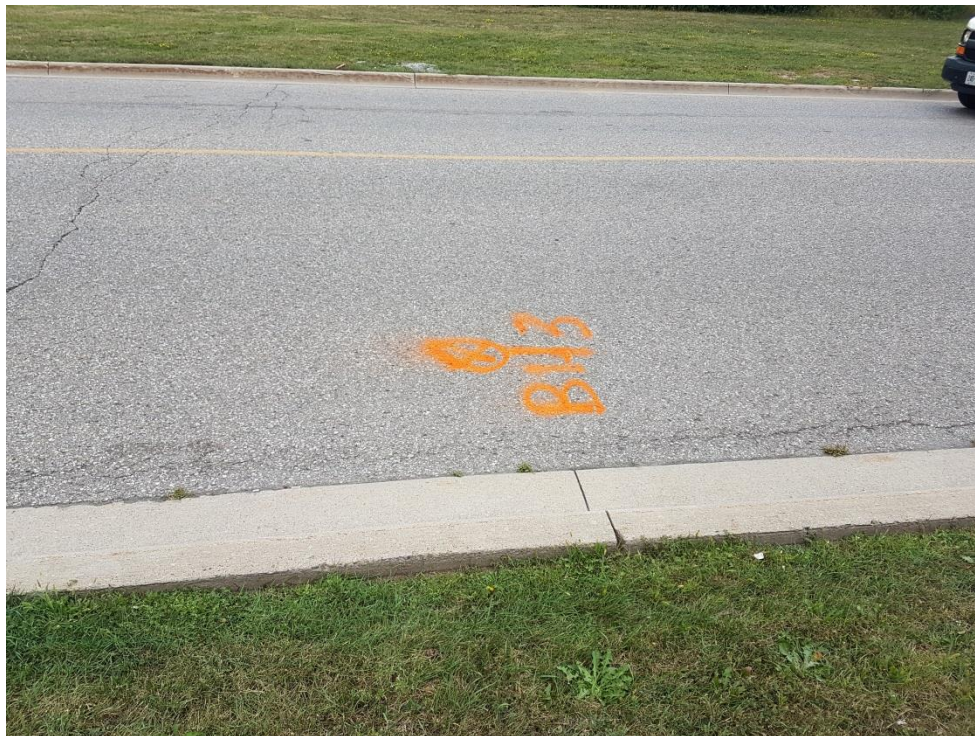
Photograph 8: Transverse and longitudinal crack near BH3 at west section of Sheridan Park Drive.
