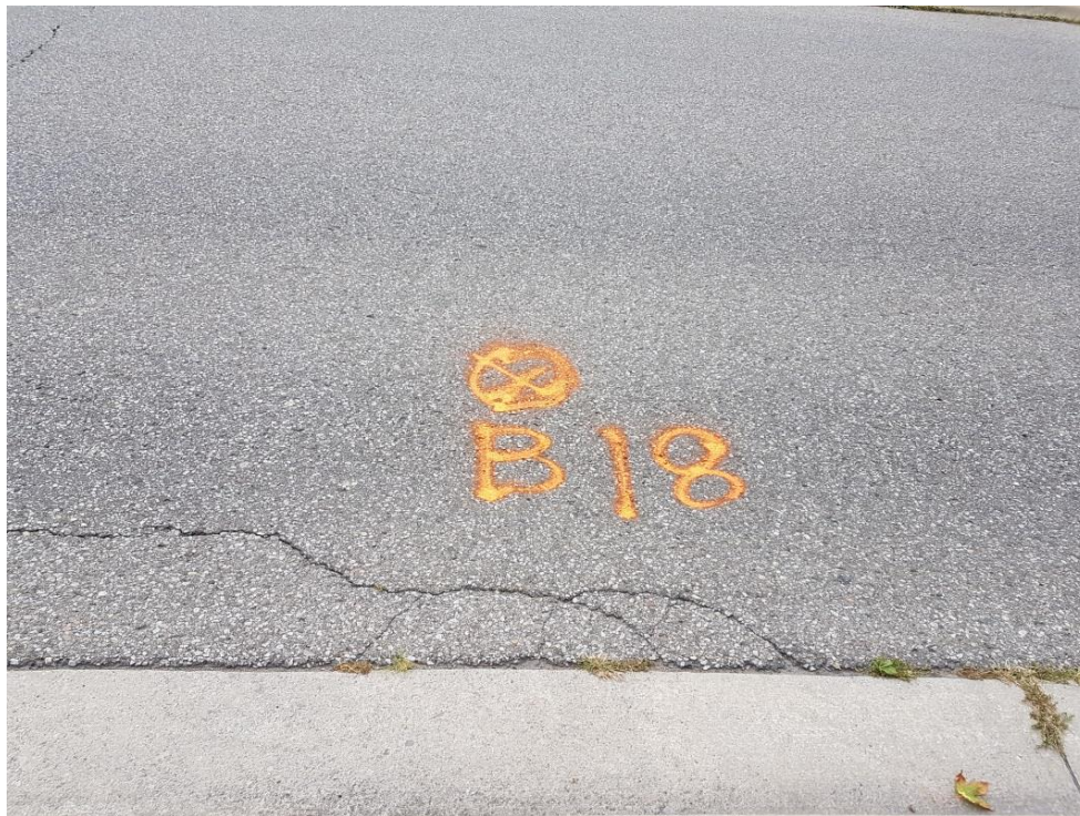
Photograph 14: Minor coarse aggregate loss and longitudinal crack along curbline near BH18.
