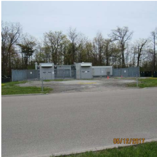
Plate 5: Southeast view of transformer facility on Sheridan Park Dr; Area is disturbed, no potential
