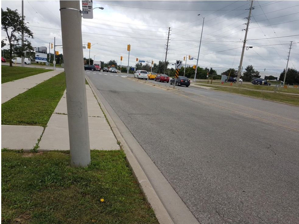
Photograph 1: Minor coarse aggregate loss and random crack near Winston Churchill Boulevard.
