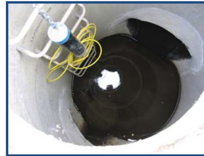
Sewer Flow Monitoring
