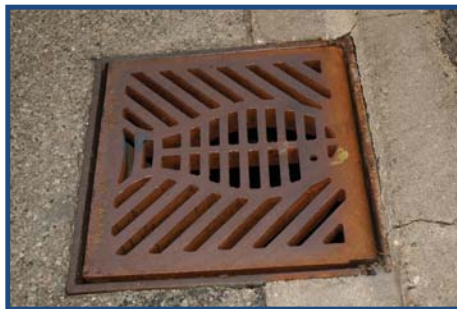
Fish-Shaped Catchbasin Grate
