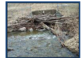
Culvert Blocked with Debris
