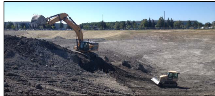
The Cooksville Creek stormwater management facility located north of Matheson Boulevard West will be the largest facility within the watershed.
