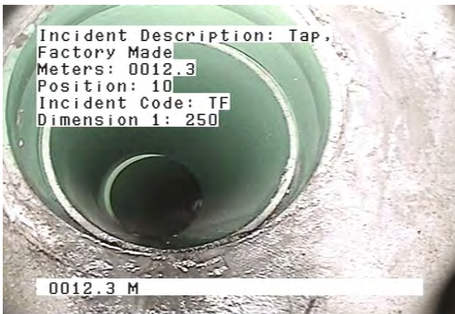
TF - Tap, Factory Made @ 12.3 m.
