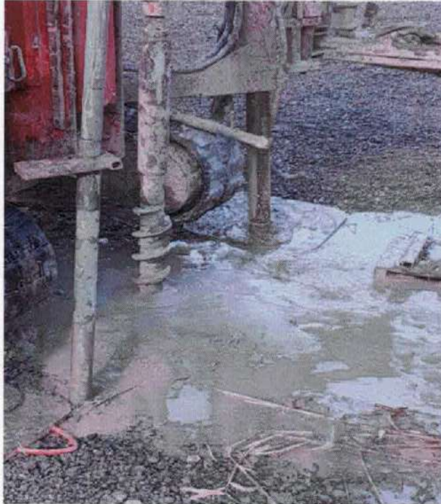
Underground water in building area, coming out from hole
