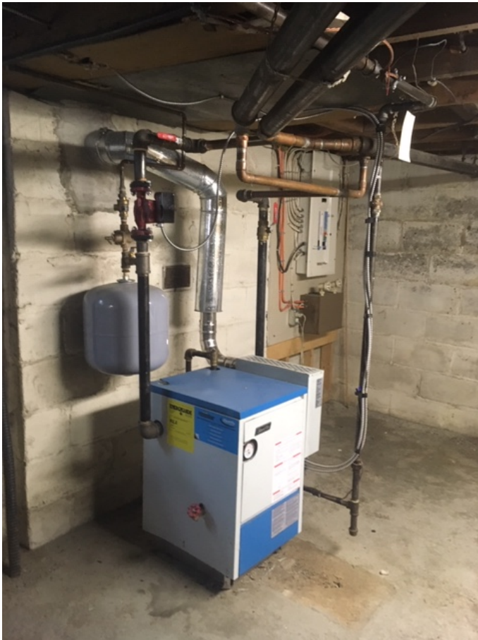
Modern Boiler in Basement
