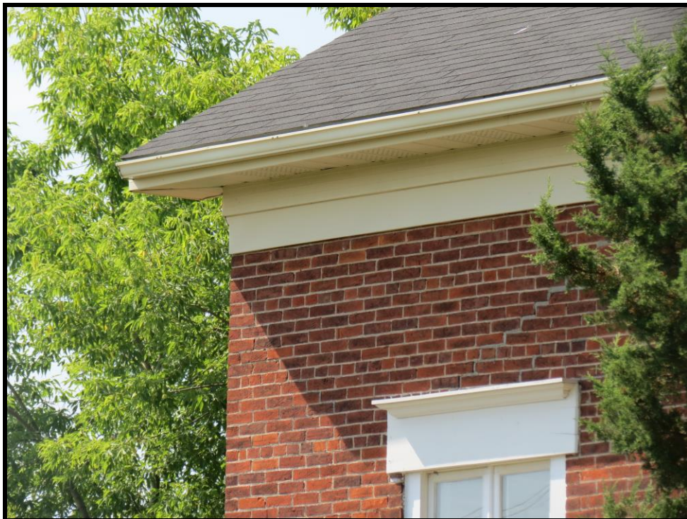
Image 24: Detailed View of Cladding, Window and Roofline, 5104 Ninth Line (Photo taken on July 29, 2019; Facing Southeast)
